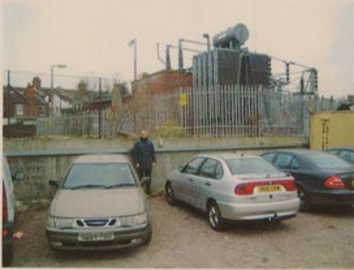
sub-station adjacent to site
